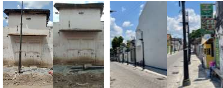
Figure 2. The installment of light pole that has not taken into account the existing building entrance, and the distance between two pole is too close.
